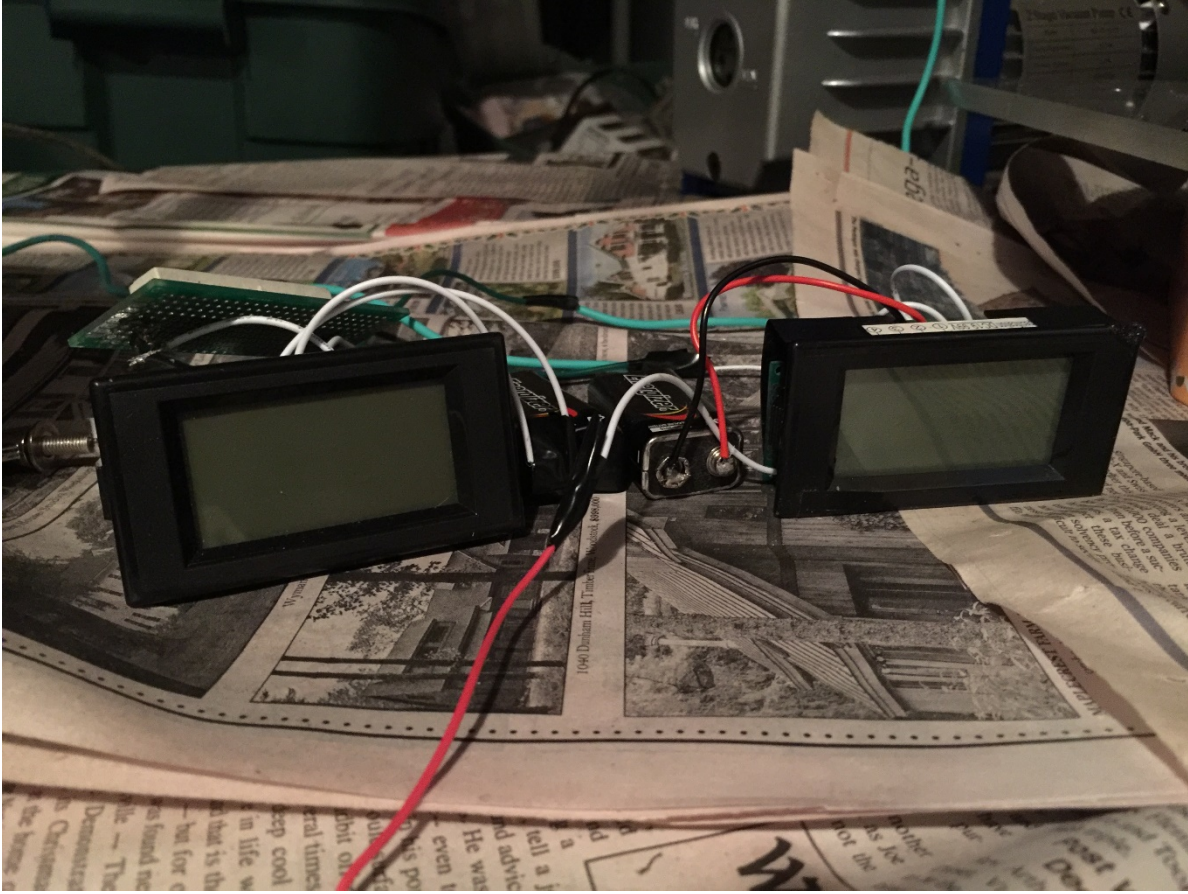
Voltage and Current Metering
